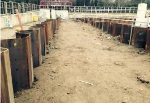
Sheet piling works have been completed with most of the plant removed from site
