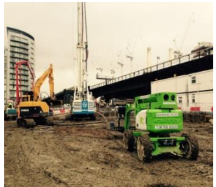
CFA piling activities is currently taking place on Block-L , having completed the all piles in Block-C
