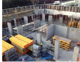
All columns on core 1 are complete and progress is on going towards Core 2
