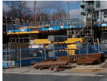
The ground floor formwork on core 1 is near completion and will be progressing on to core 2
