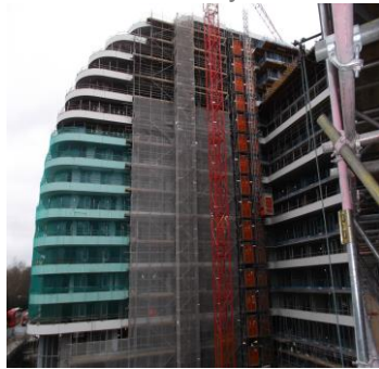
Block C is now at level 15 and the roof has been cast.
