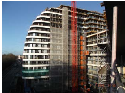
Block C is now at level 15 and the roof has been cast.
